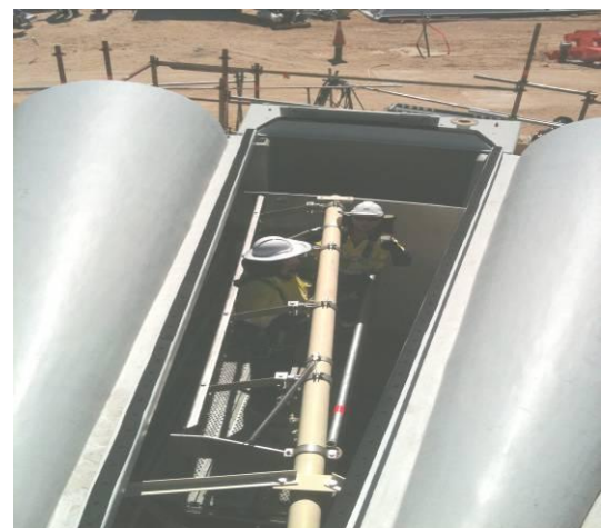
Working in confined space, post JHA and implementation of risk and control system
